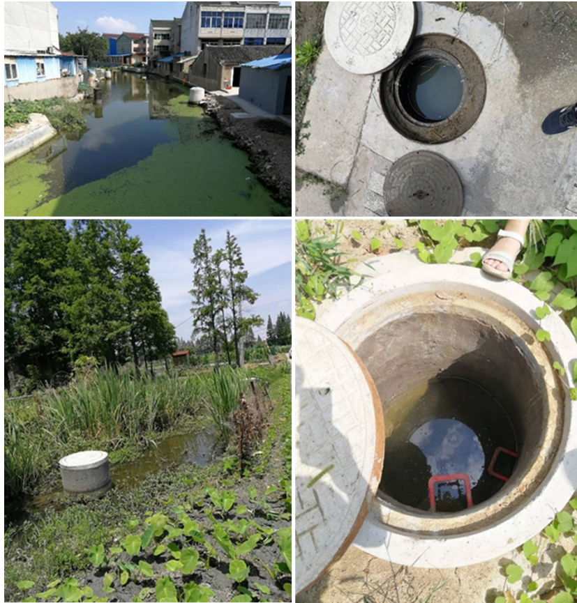
Fig S4. Digital photos of pipe network for transporting rural sewage. Most of the pipe networks were built closing to low-lying places, irrigation canals and ditches even rivers, therefore showing high risks of leaking.
